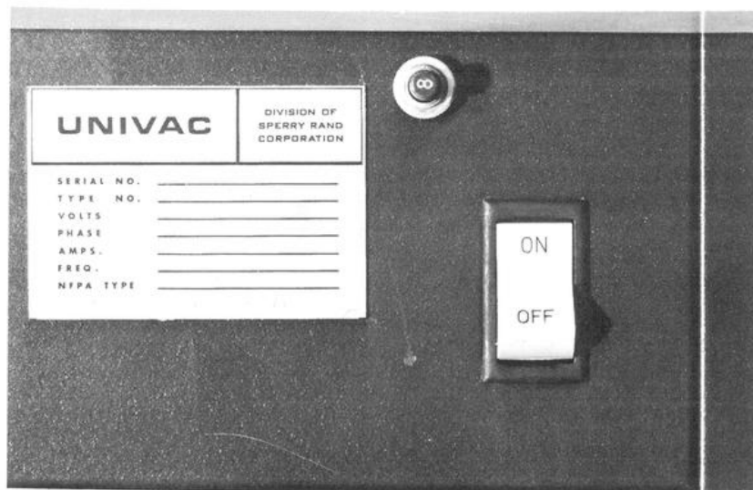
The Power Switch with the Circuit Breaker just above it.
